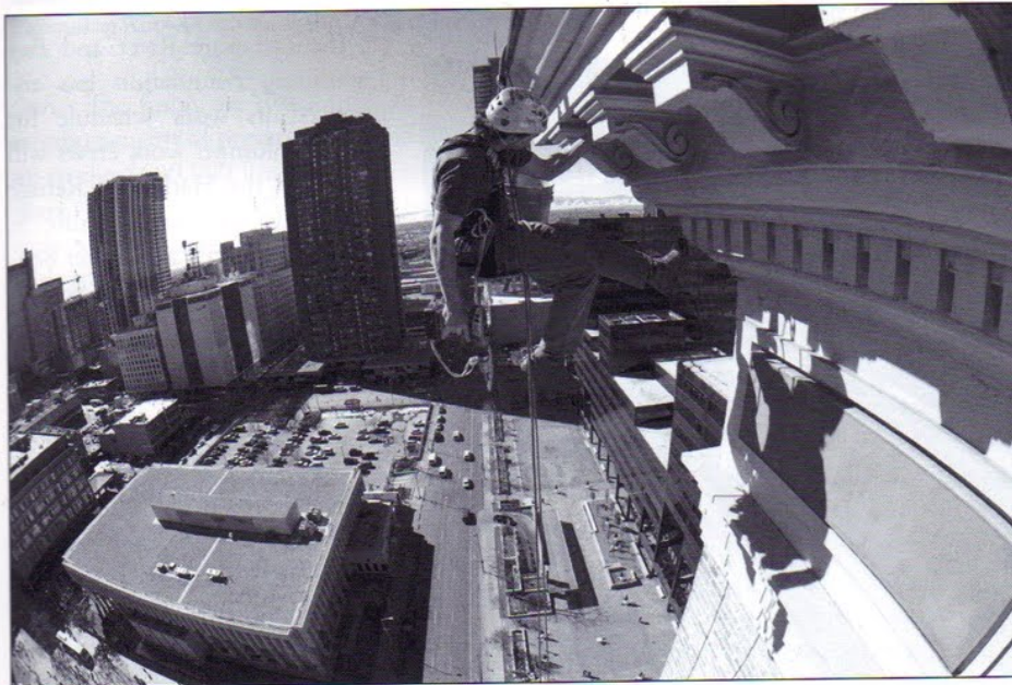
A worker dangles above the city skyline while working on decorative roof brackets. Photo courtesy of Rich Purnell of the BASE Group.
